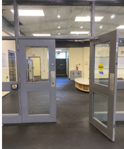
Automatic door openers at Frank Crane Arena
