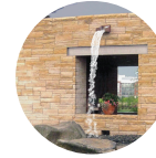
09 Wall Scupper: overflow water from the upper raingarden flows through a scupper in the retaining wall to the lower raingarden
