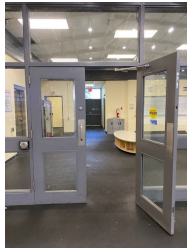
Automatic door openers at Frank Crane Arena
