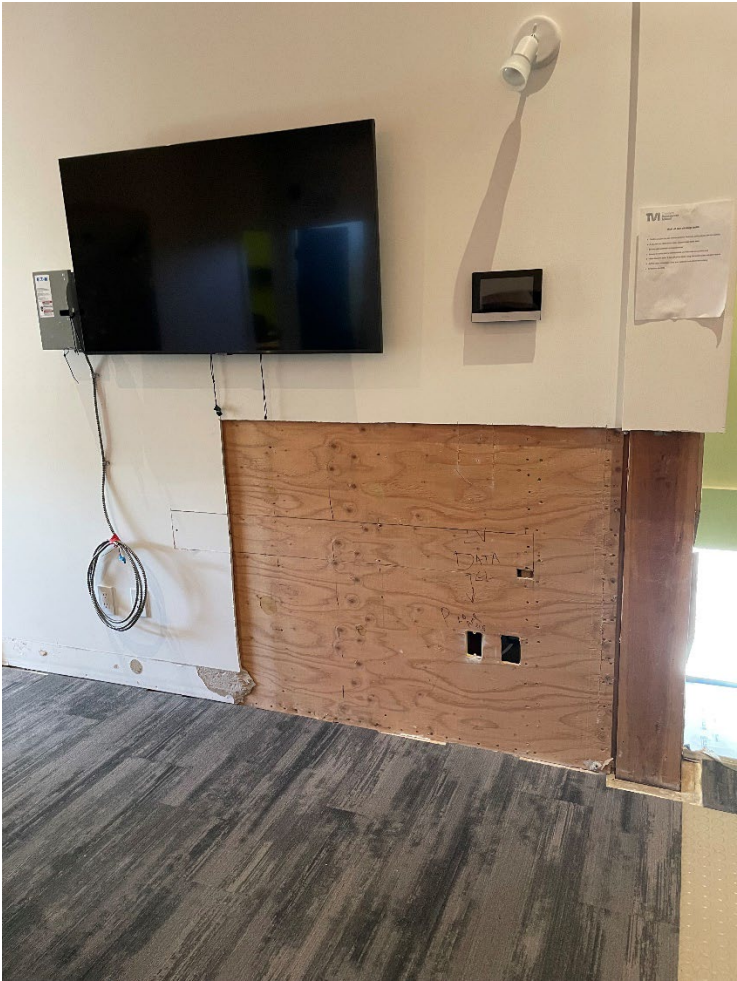
Lift House Box & Electric Panel
