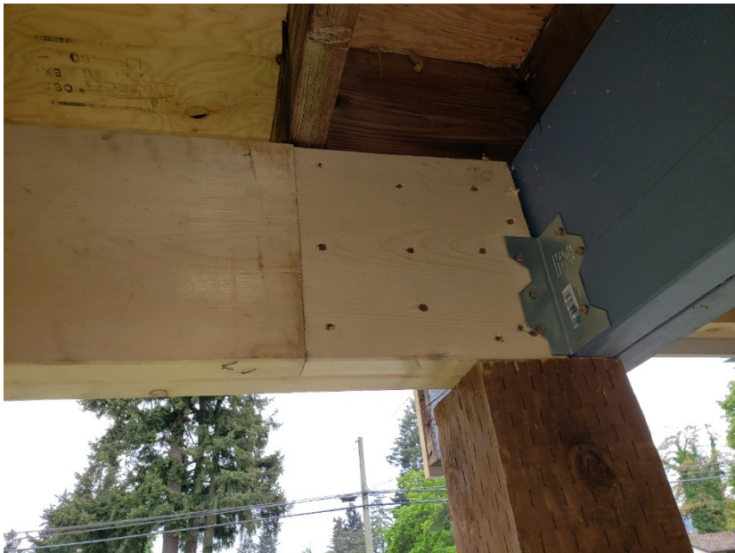
2-ply beam spliced incorrectly with deck screws.
