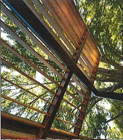
4 Trellis - Black Metal Post and Wood Purlins _____
