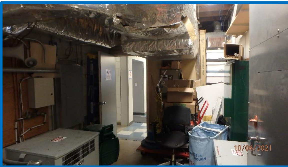
Image 20 Inefficient Heating and Cooling
