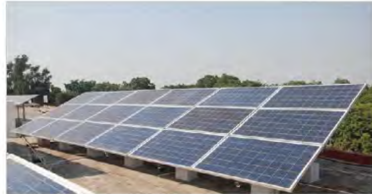
Rooftop PV system
