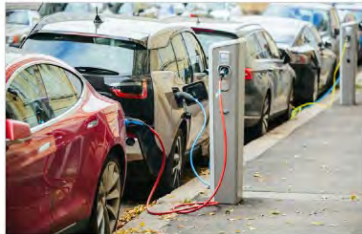
Electric vehicle charging stations
