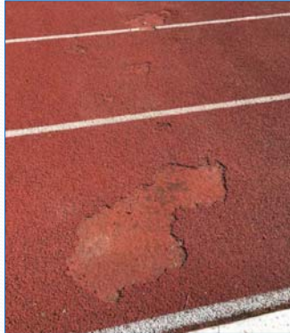
Track surface damage
