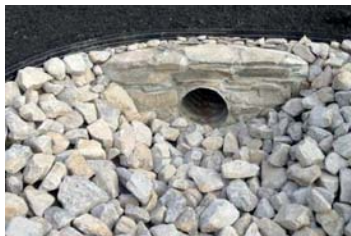
Armoured Swale Photo
